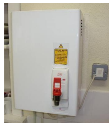
Hot water boiler
