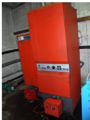
Stand-alone centralised water heater
