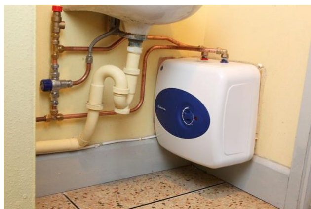
Local electric water heater
