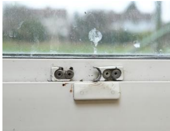
Broken window latch
