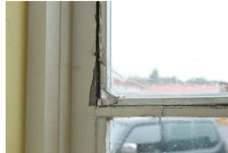
Deterioration of internal window frame
