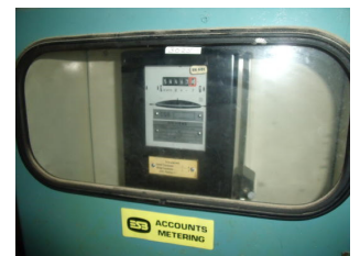
Meter and ESB Enclosure
