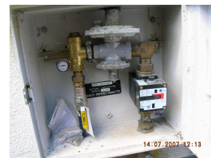
Meter inside cabinet
