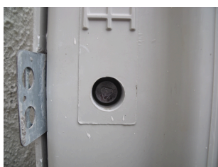
Meter cabinet keyway
