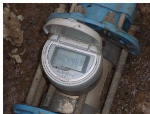
Large Water Meter
