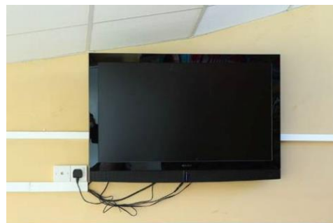
Make sure sockets controls are within easy reach.
