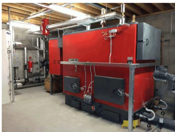
Biomass boiler in pilot school
