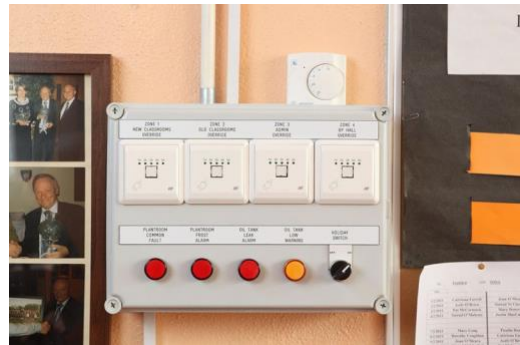
Zone heating manual over-ride controls panel
