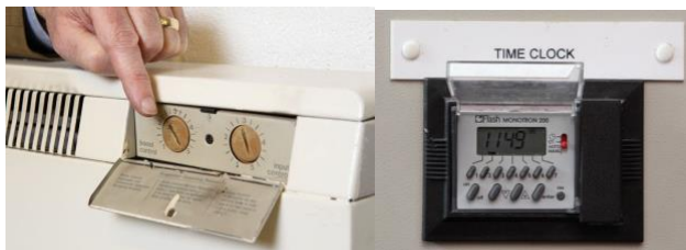
Typical Storage Heating Controls (left) and 7-day time-clock (right)
