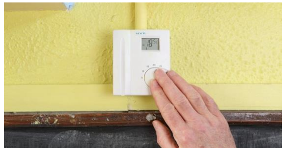
Typical Room Thermostat in School
