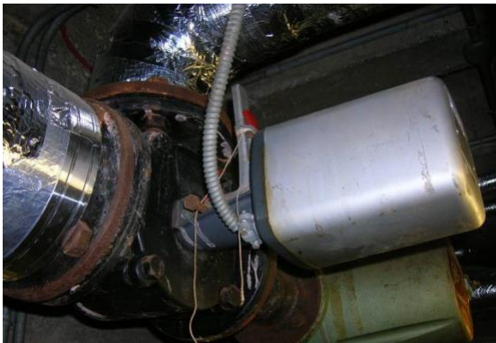
This is a weather compensator valve that has been disabled with a piece of string. As a result, the schools fuel bills will be up to 10% higher.
