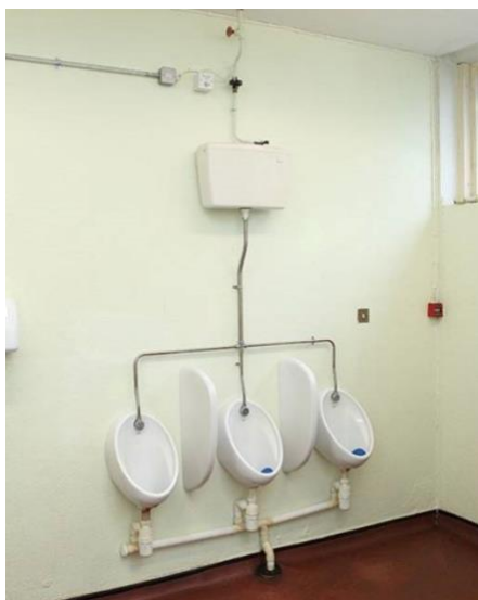
Fit urinals fitted with automatic urinal control valves to conserve water
